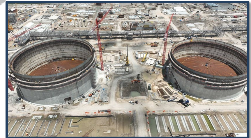
Tanks 1 and 2, June 2025
