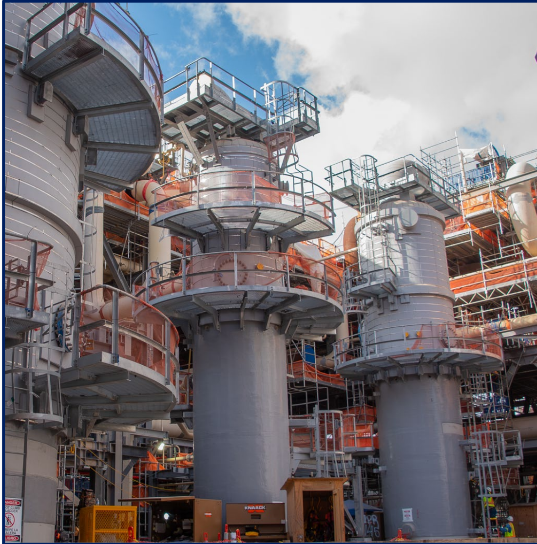
Train 1 Process Equipment, April 2026
