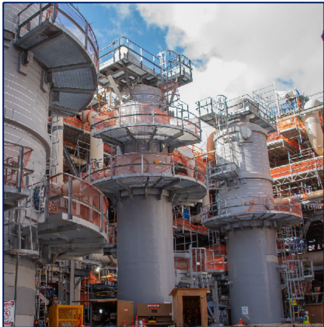
Train 1 Process Equipment, April 2026
